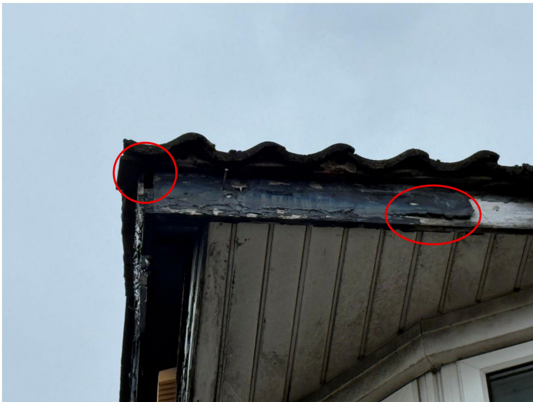
Photo 10: Gap and delaminating fascia board on eastern elevation of building B3.
