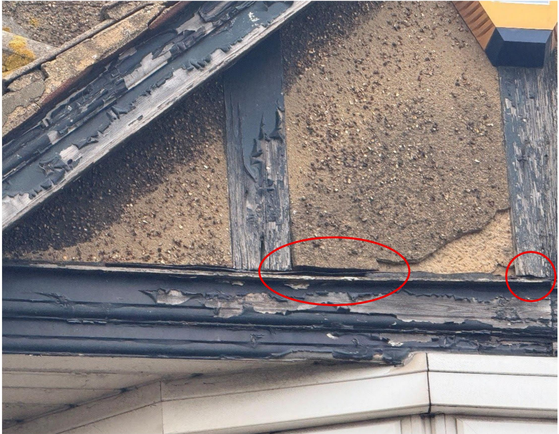
Photo 11: Delaminated render and lifted timber on building B3.
