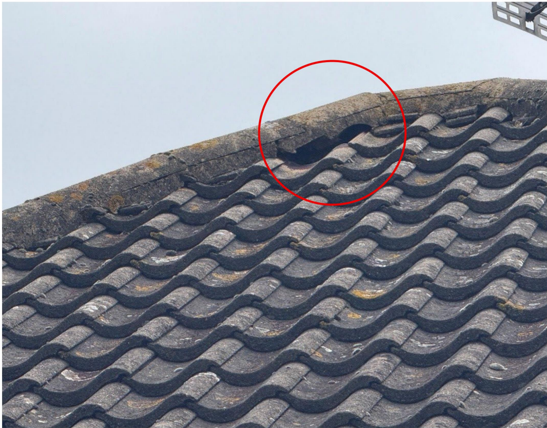
Photo 9: Missing tile leading to internal cavity on building B3.
