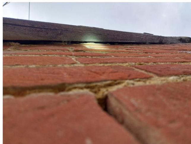
Photograph 12: Gap between bargeboard and wall on B2.
