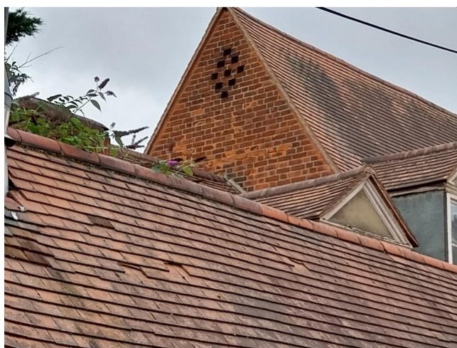
Photograph 15: Example of missing tiles and loft vents on B1.
