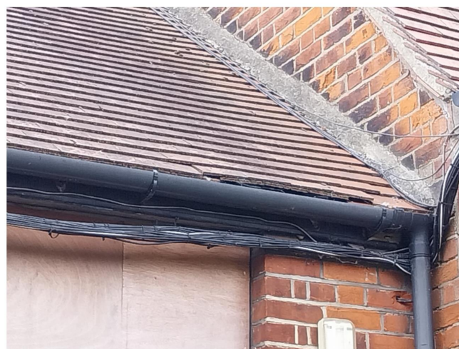
Photograph 16: Example of lifting tiles and boarded windows with gaps on B1.
