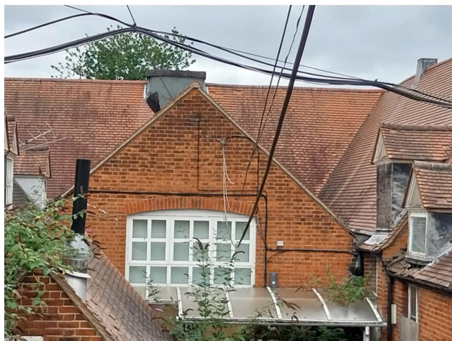
Photograph 17: Back of B1 showing missing tiles, dormers with gaps around them and lifting flashing.
