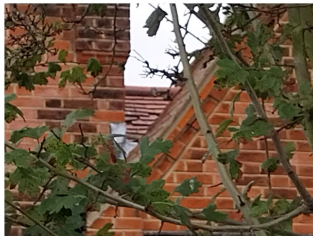
Photograph 18: Example of lifted tiles found on the front face of B1.
