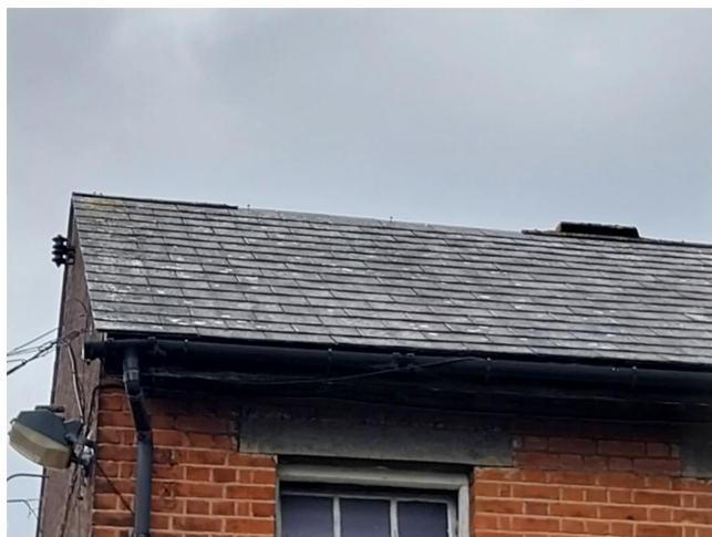
Photograph 11: Missing ridge tiles on B3.
