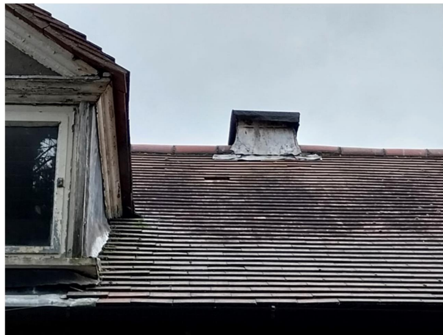
Photograph 14: Example of lifted flashing, missing tiles and dormer on B1.
