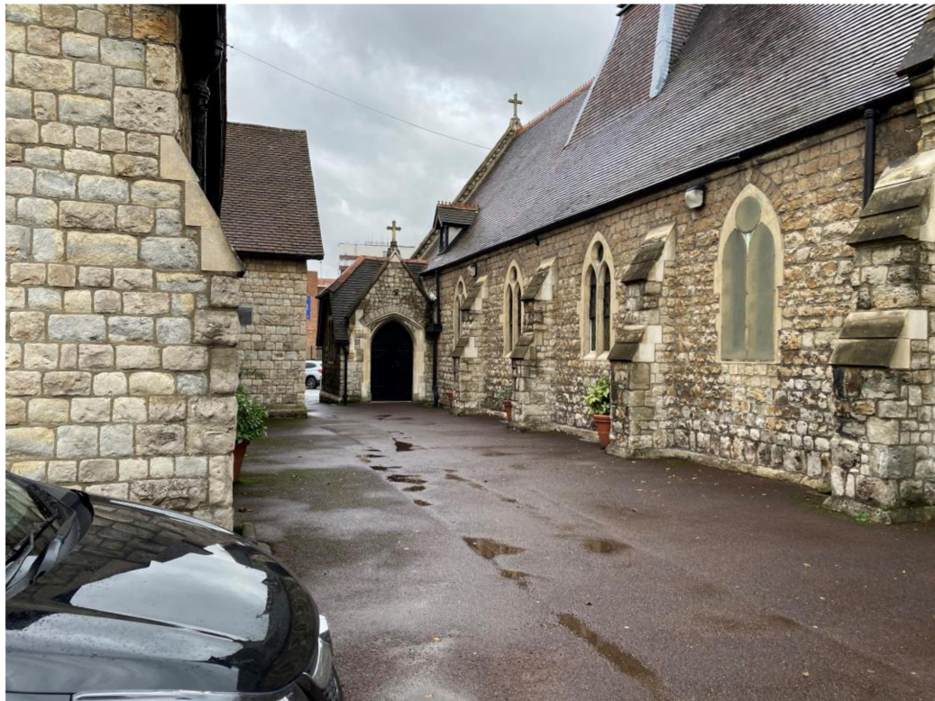
Figure 22: Gap between the church and former school (left)
