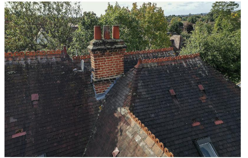
(D) Existing Roof view including decorative ridge detail
