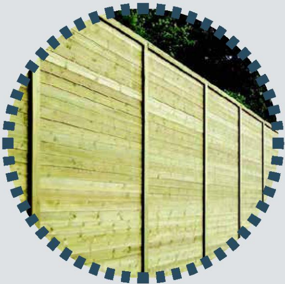
Jacksons Acoustic fencing 2m high above podium. Total height from yard level is 7m.
